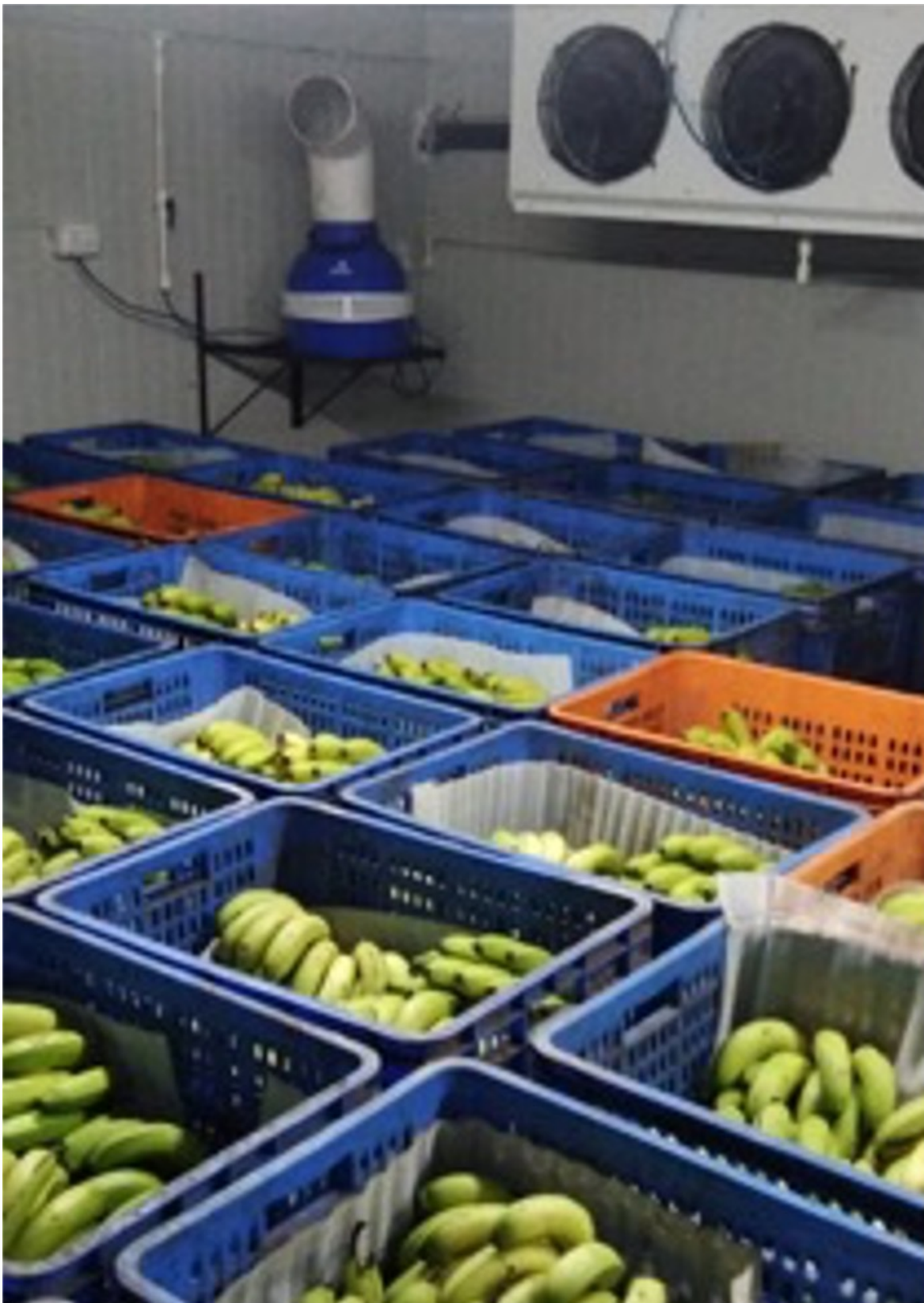
Industrial ripening chamber with refrigeration and gas control (Credit: Nilkamal)
