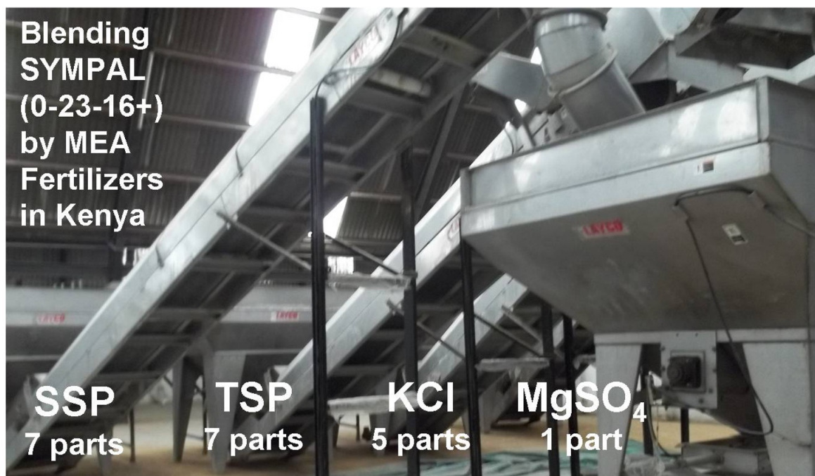
A multichannel blender in operation at MEA Fertilizers used to produce SYMPAL for grain legumes in Kenya
