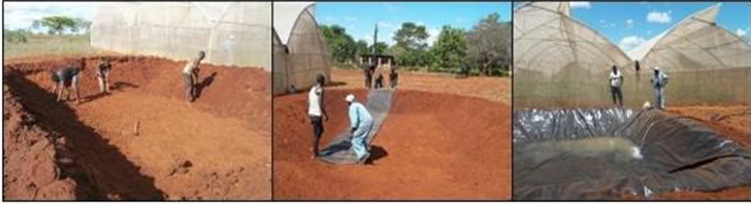
Establishing a small fishpond (left to right): 1) excavating and smoothing the pond, 2) spreading the PCV liner and burying the edges, and 3) filling the pond
